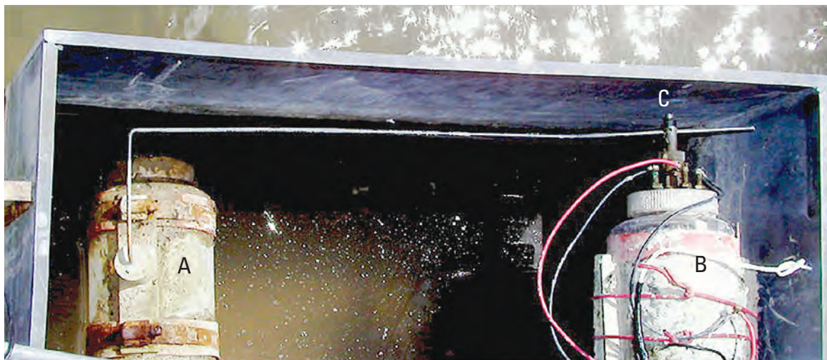
Figure 2. Photograph of the interior of the stilling well box showing the float gage. A, The bottle at the left is a float that is connected to the precision wire-wound potentiometer contained in the bottle to the right. B, The shaft of the potentiometer. C, is sealed by an O-ring where it passes through the bottle cap. This seals the interior of the bottle from the atmosphere. However, over time, a small amount of water enters the bottle. This leakage is captured by silica-gel desiccant contained in a cloth bag inside the bottle. The stilling well box is covered to prevent snow buildup on the equipment.
