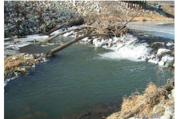
Downstream view of Seven Mile Creek water control weir before structure modification.
