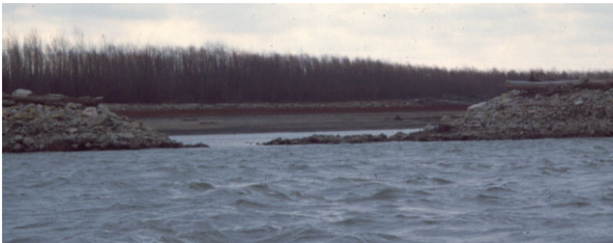
Example of a deep notch on an L-dike that allows scouring flows at normal water stages
