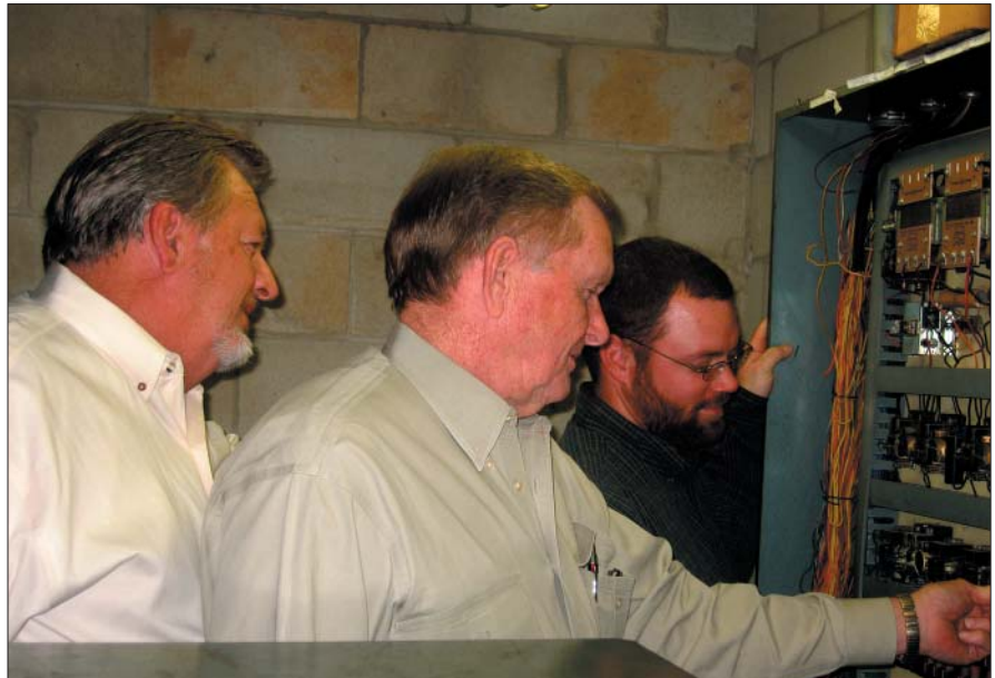
The Arkansas Department of Labor and small business owners worked closely in revising state elevator regulations. Pictured here are James L. Salkeld, director, and Larry Smothers, chief elevator inspector, Department of Labor; and Clayton Billingsley, co-owner, Tri-B Realty Inc.
