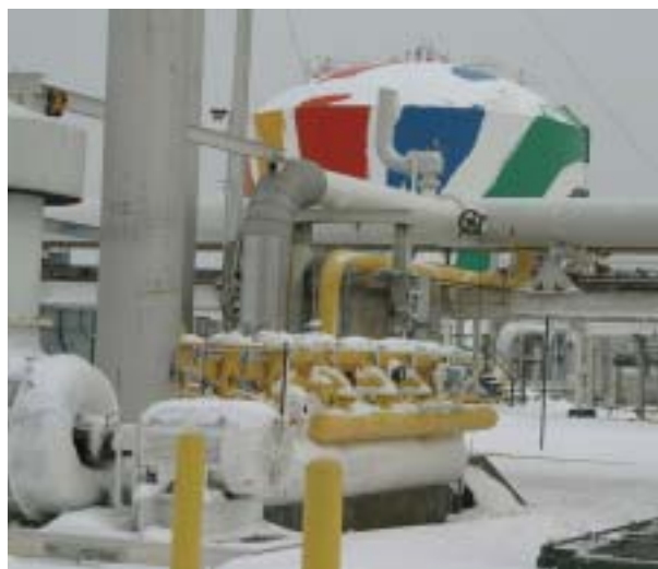
Figure 4 Peak-shaving facilities make LNG from pipeline gas during peak periods of low gas demand and store it until it is needed.
