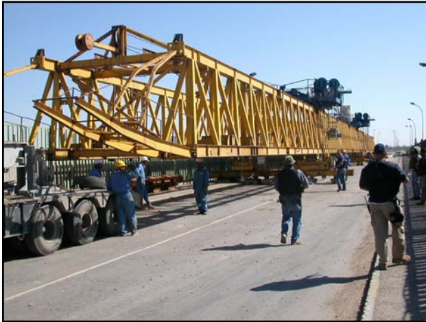
Tikrit Bridge beam launcher re-positioning. Traffic currently crosses the Tigris at this point over a two-lane temporary bridge. Opening the four-lane Tikrit Bridge will improve passenger and commerce traffic.
