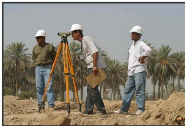
Iraqi civil engineers working in Baghdad, survey the site preparation for an extension to the Saba Nissan water Treatment plant as part of a grant to expand drinking water for the Baghdad region. (Photo: Thomas Hartwell)
