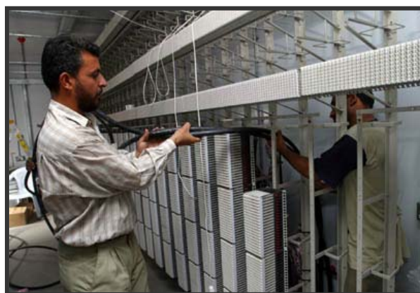
The Al-Mamoun Telephone Exchange where repair work will restore telephone services to approximately 30,000 subscribers. (Photo: Thomas Hartwell)
