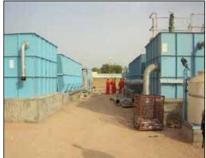
Compact water treatment units at the Karbala water treatment plant
