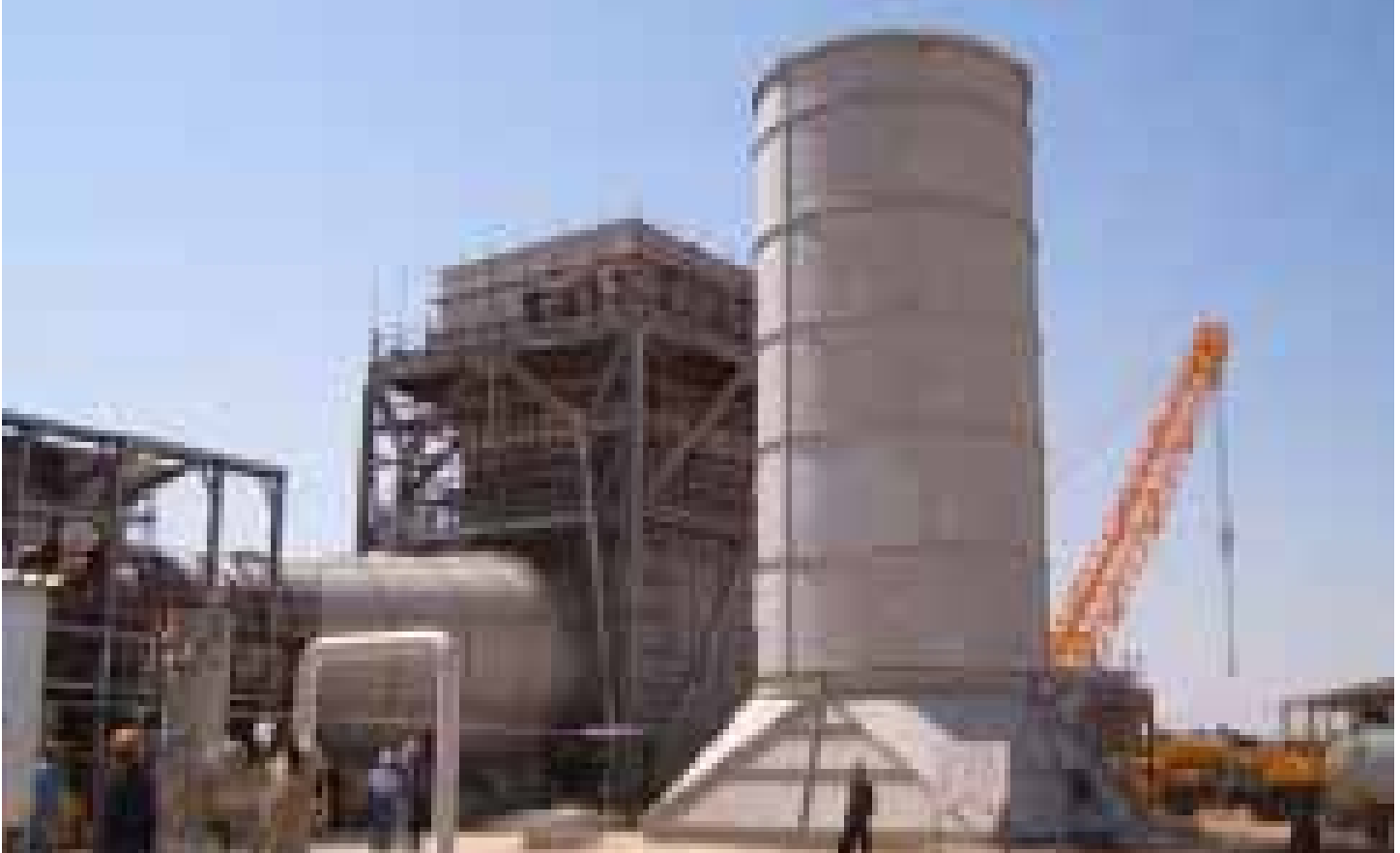
Combustion turbine and exhaust stack at the Taza substation in Kirkuk. Work at the substation will add 325MW to the national grid upon completion.
