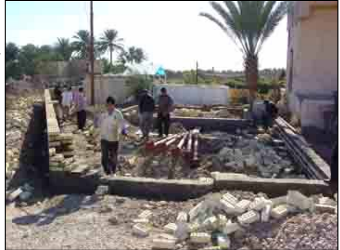
Villagers in a rural community outside of Baghdad prepare pipe installations to rehabilitate the village potable water station.
