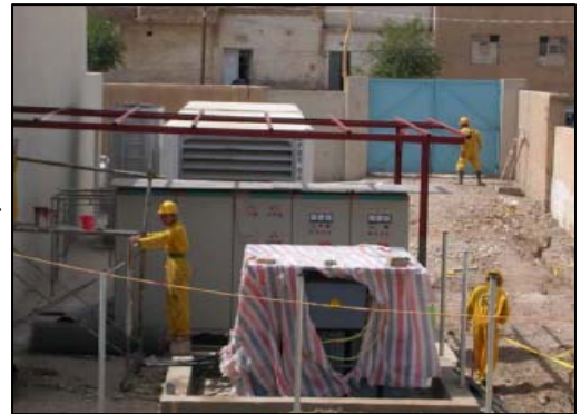
Repairs to water and sewage treatment plants in the Diyala governorate near completion. These plants will supply clean, potable water to a community of 60,000 residents.
