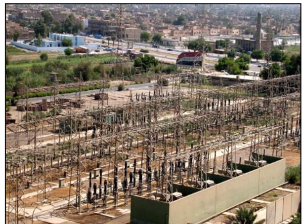
Baghdad's Doura power plant. USAID Photo.
