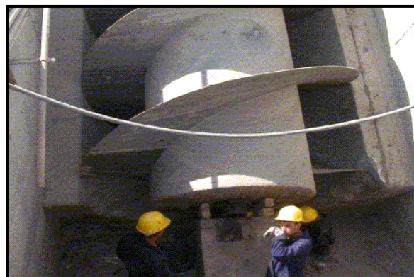
Repaired Archimedes screw, which helps move the water up to the beginning of the treatment process
