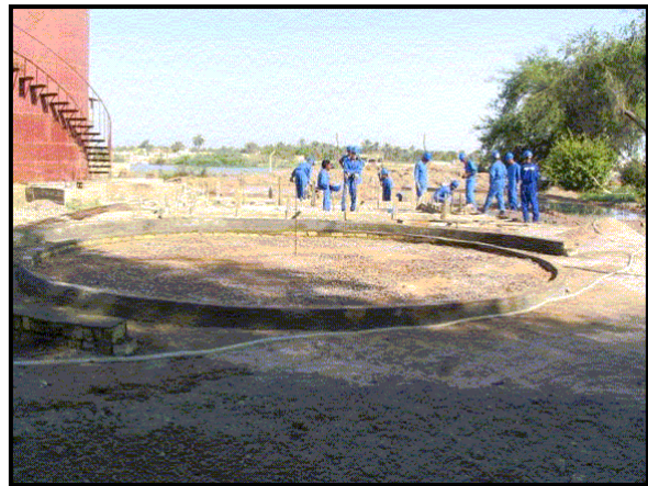
Foundation for a water treatment unit at a thermal power plant in southern Iraq
