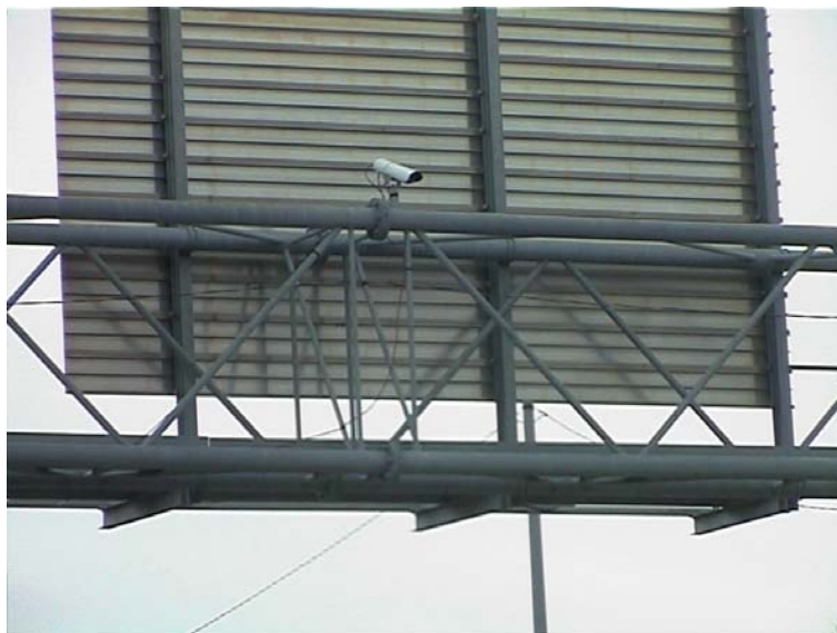
Figure 3. WZSAS Camera Mounted Above Roadway
