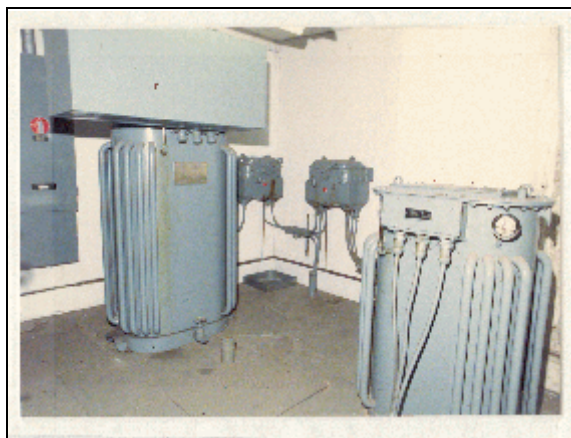
Figure 4-1. Two PCB Transformers.
