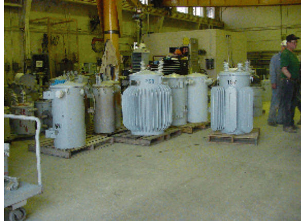
Figure 3-3. PCB Transformers in storage.
