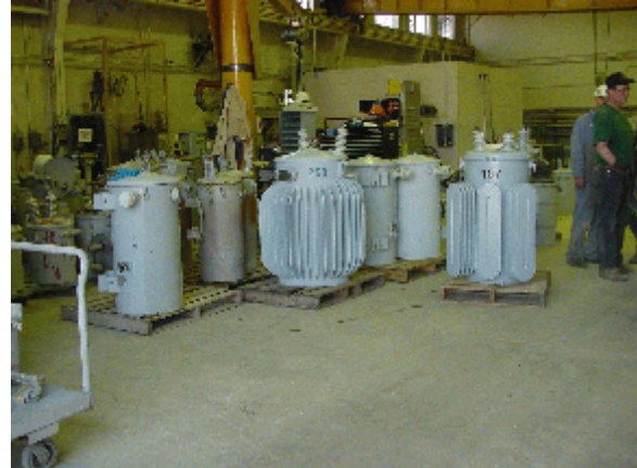
Figure 2-3. PCB Transformers in storage.
