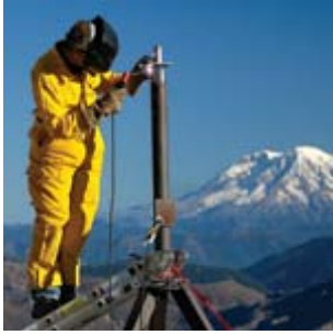
An EarthScope worker welds a GPS station on the flanks of Mount St. Helens. Such stations will precisely monitor deformation associated with magma movement within the volcano. Credit: EarthScope.
