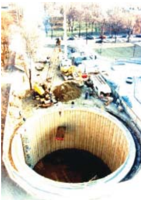
Figure 13. Secant piles used for excavation and wall construction in the Trevipark (from the TREVI Group presentation).
