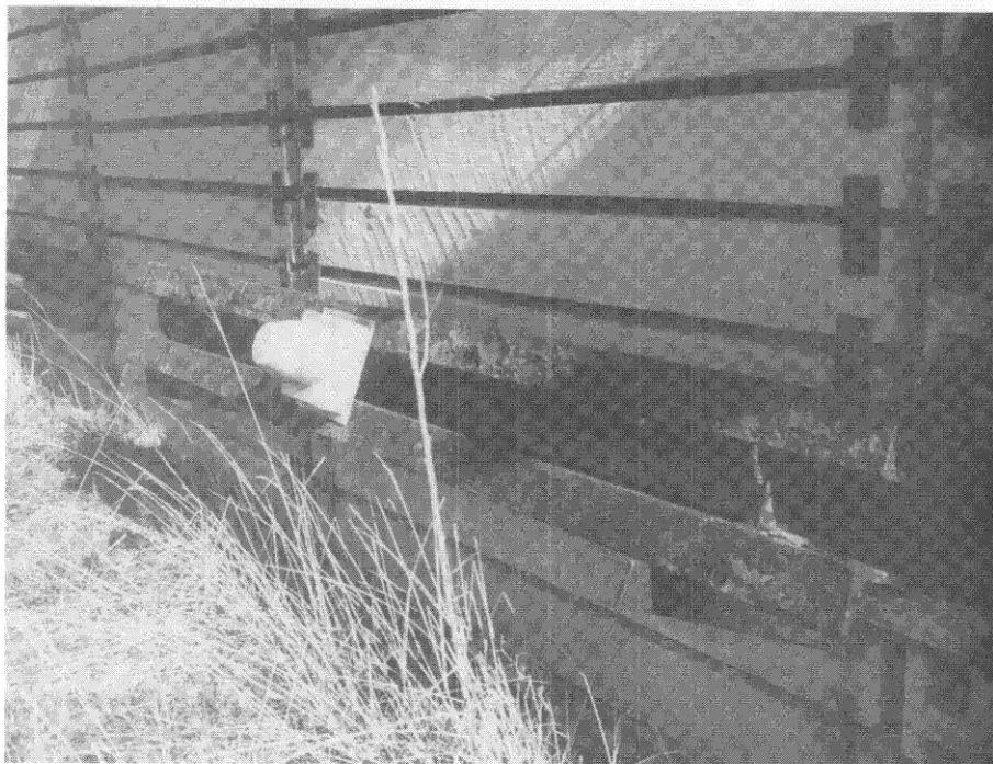
Figure 6E Blistering and Peeling of Protective Coating on Waler
