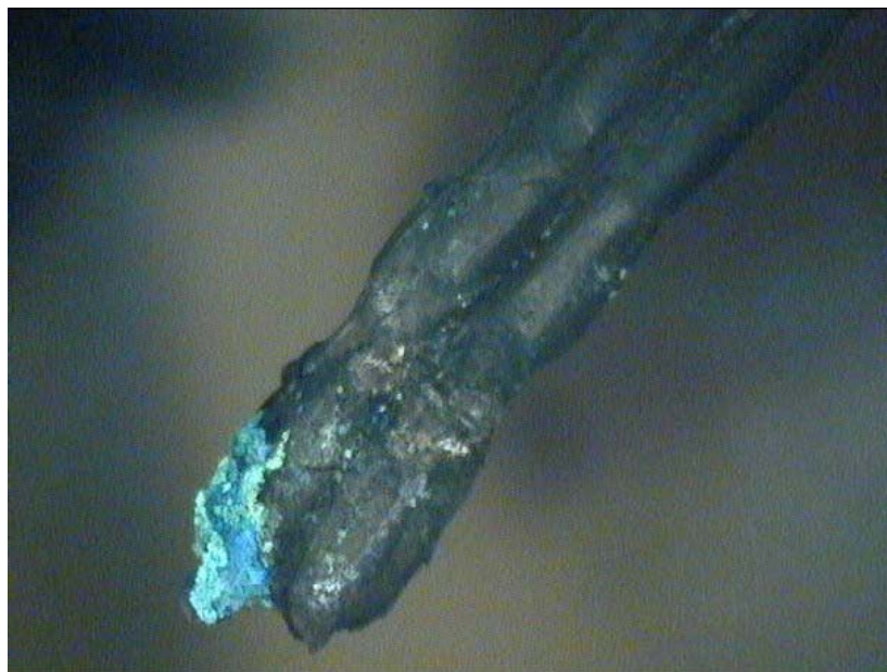
Figure 14. Electrical Wiring in Socket
