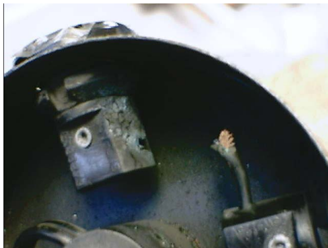
Figure 6. Damaged Fourth Socket of Incident Sample
