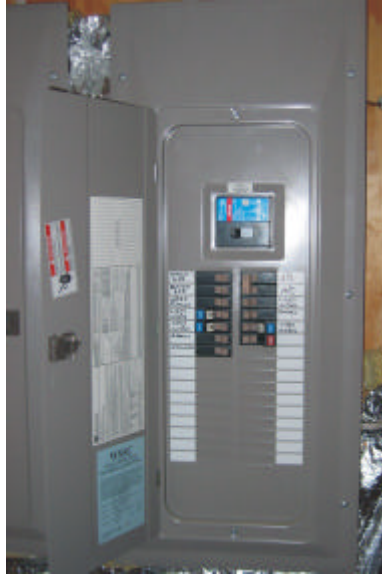
Figure 5. Example of Panel Board with Circuit Breakers
