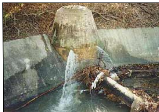
SSOs contain human waste and other debris, such as toilet paper.
