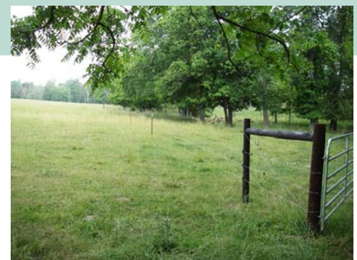
Livestock exclusion fencing was installed to protect the riparian zone along Cooper Branch.
