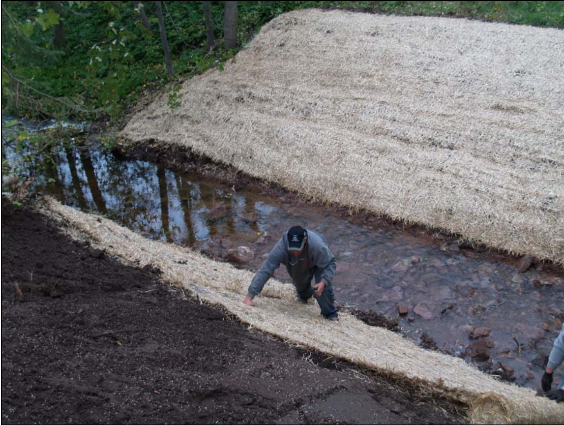
Figure 6-2. In 2007, a grant from US EPA Great Lakes National Program Office allowed the Superior Watershed Partnership, Upper Peninsula Resource Conservation and Development Council, and Michigan Waterfowl Association to remove the culvert and stabilize the banks of Orianna Creek.
