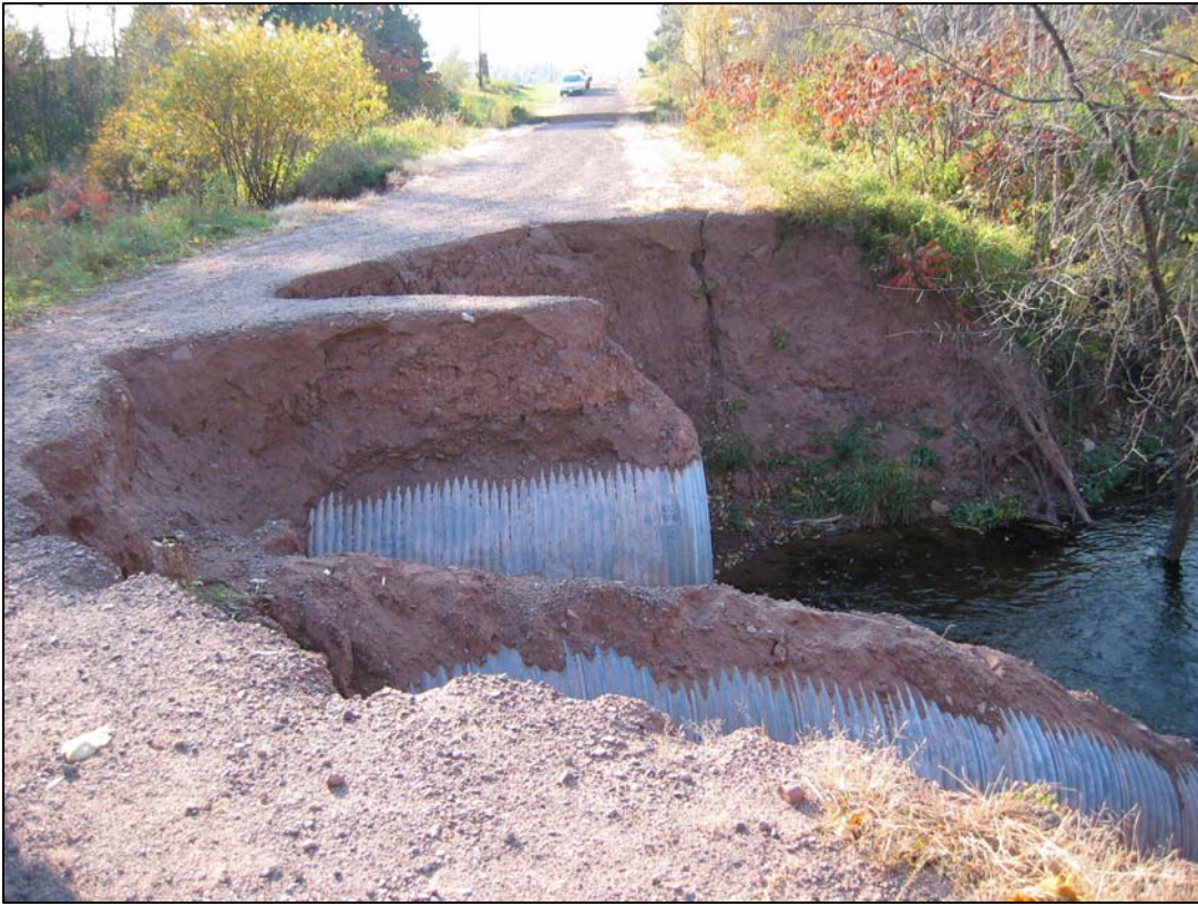
Figure 6-5. Silver Creek culvert failure in 2003. Photo credit: S. Schultz, Stable Solutions LLC.
