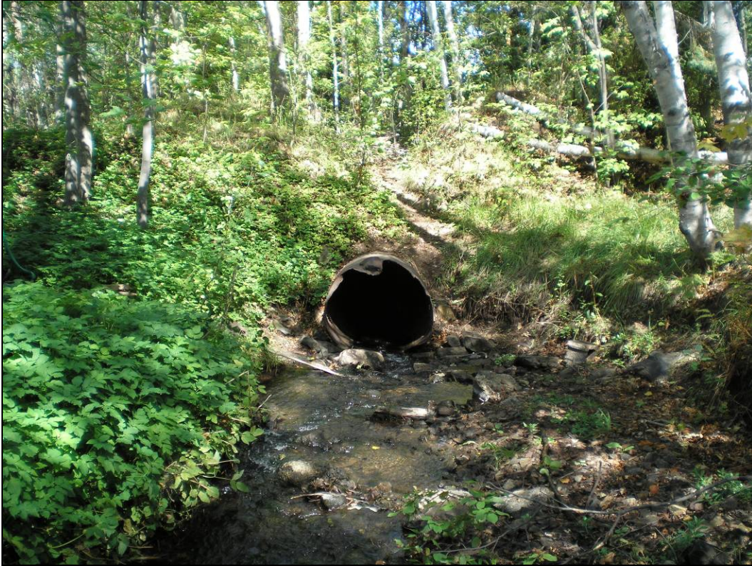
Figure 6-1. Watershed management plans lead to restoration actions. The Whetstone and Orianna Creek Watershed Management Plan for Marquette, Michigan, identified this old abandoned culvert on the Orianna Creek as causing erosion and sedimentation to the stream, as well as being a barrier to fish passage. Photo credit: Superior Watershed Partnership.
