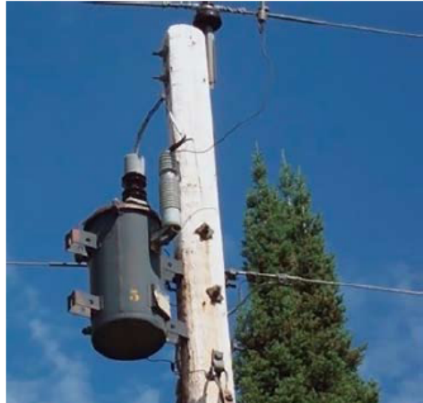
A PCB transformer. Photo Credit: Scott Bohling, Minnesota Pollution Control Agency.
