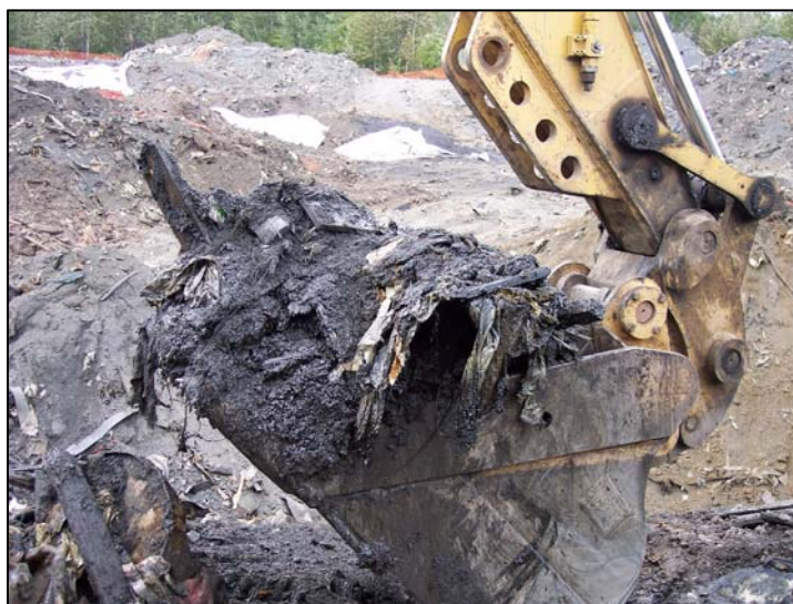
Figure 4-11. Oily debris from the Reserve Mining barrel dump site in Silver Bay, Minnesota. Photo credit: Susan Johnson, MPCA.
