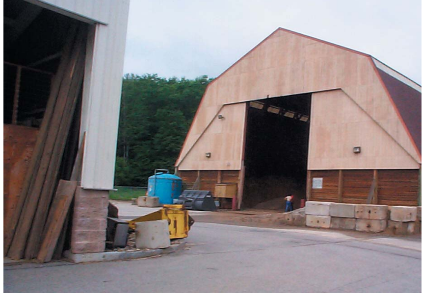
Building sheds to cover sand/salt mix, roofing refueling operations, and simply keeping dumpster tops closed are ways municipalities can insure that storm water runoff is not harming their drinking water wells or surface water resources.
