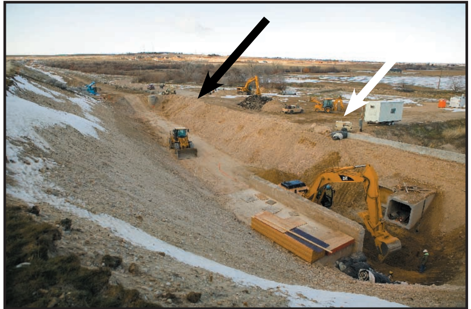
Repairs to the outlet at the Nampa Canal. The black arrow indicates the abrupt end of Lake Avenue, and the white arrow indicates the usual boat ramp overflow parking lot (photo copyright Mike Shipman).
