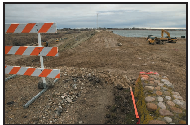
View east along the Upper Dam across the breach where the Caldwell Canal is being repaired (photo copyright Mike Shipman).
