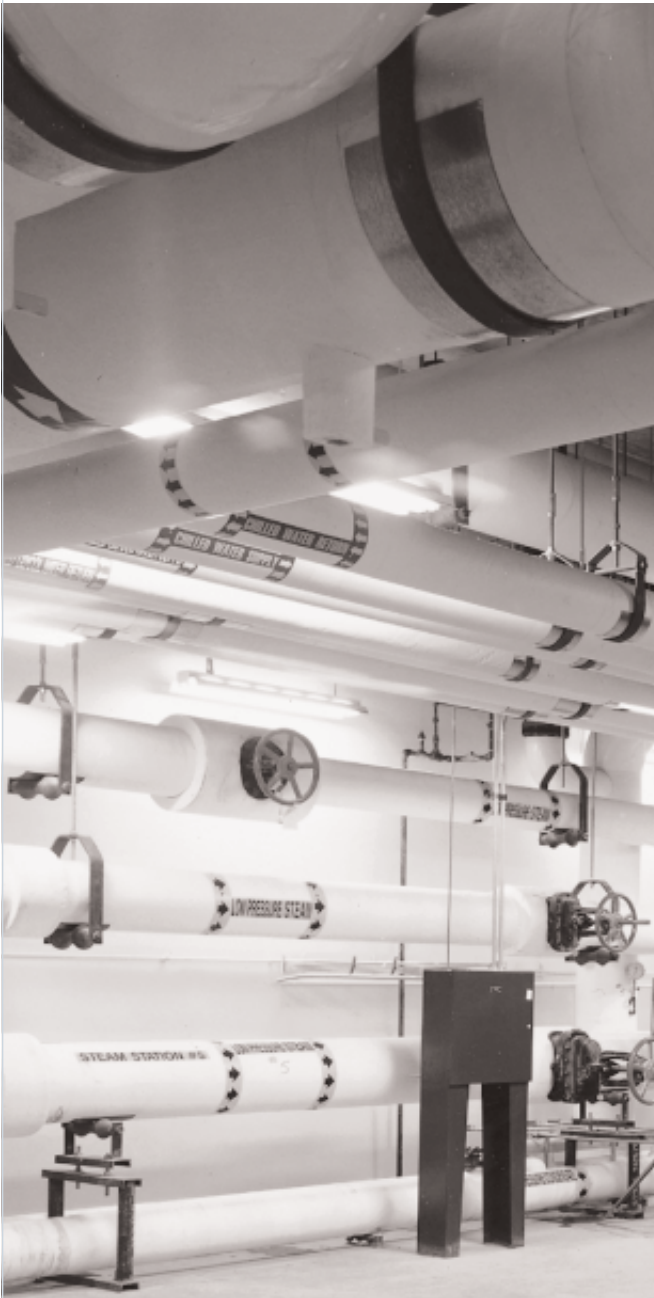
College Park, Maryland chilled water supply and return
