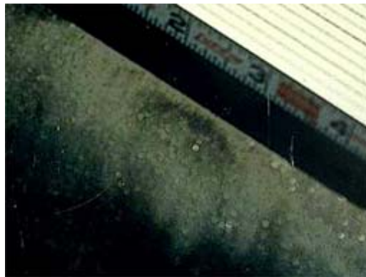
Figure III-5. Pipeline Defect (Wall Thinning Due to Corrosion)
