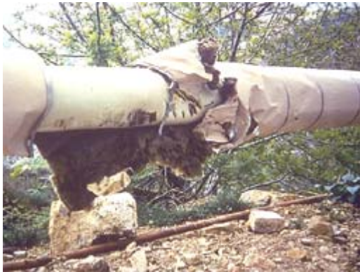
Figure III-1. Above Ground Pipeline Damage
