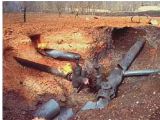
Figure III-2. Pipeline Rupture from Outside Force
