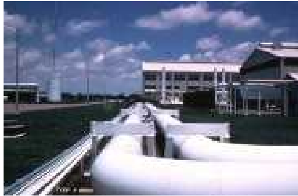
Figure IV-5. Unpiggable Lines at a Compressor Station
