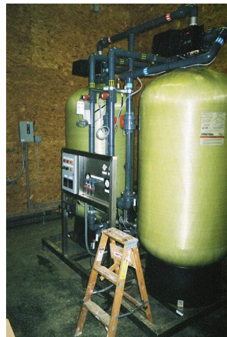
Rollinsford's new arsenic water treatment equipment
