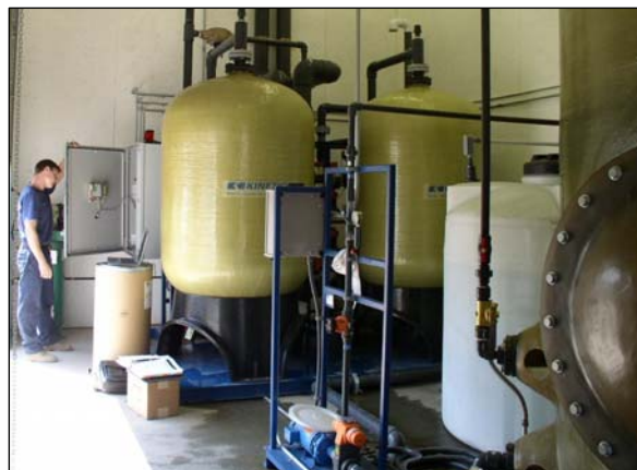
Fruitland's new arsenic water treatment equipment
