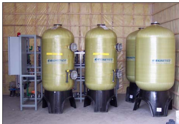
Climax's new arsenic water treatment equipment
