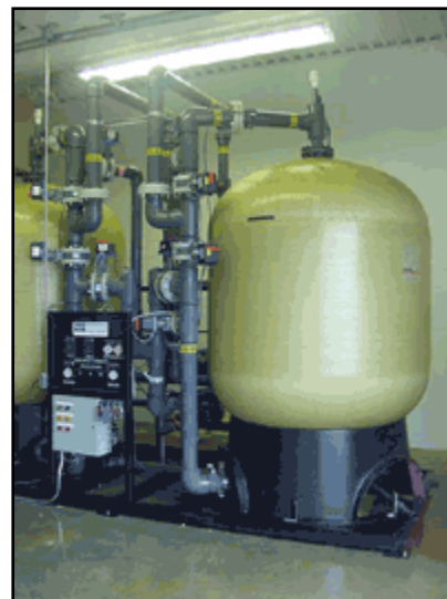
Brown City's new arsenic water treatment equipment
