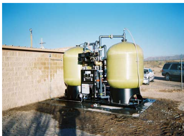
Desert Sands' new arsenic water treatment equipment
