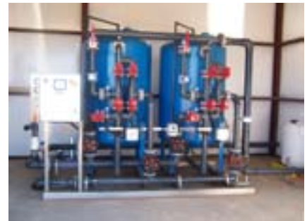
Wellman's new arsenic water treatment equipment
