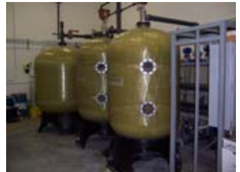
Three Forks' new arsenic water treatment equipment
