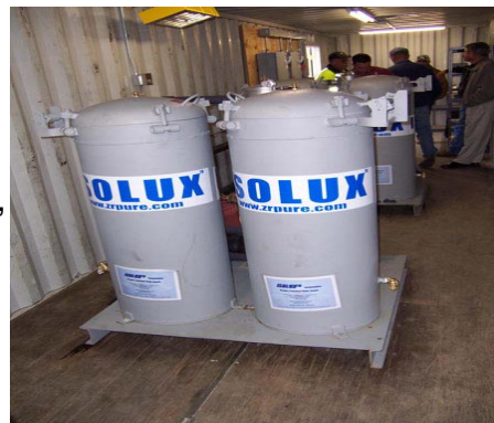
Golden Hills' new arsenic treatment equipment
