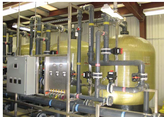
Taos's new arsenic water treatment equipment
