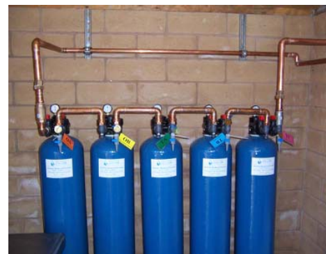
Richmond School District's new arsenic water treatment equipment
