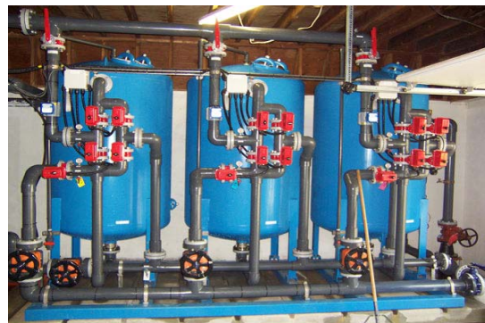
Chateau Estates' new arsenic water treatment equipment
