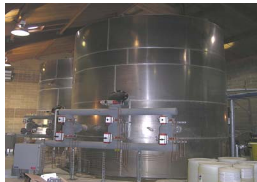
Sandusky's new arsenic water treatment equipment
