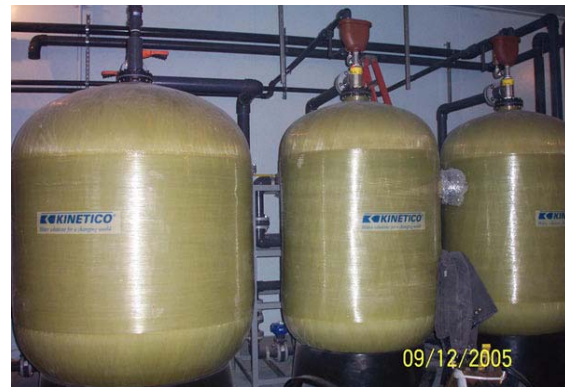
Sabin's new arsenic water treatment equipment
