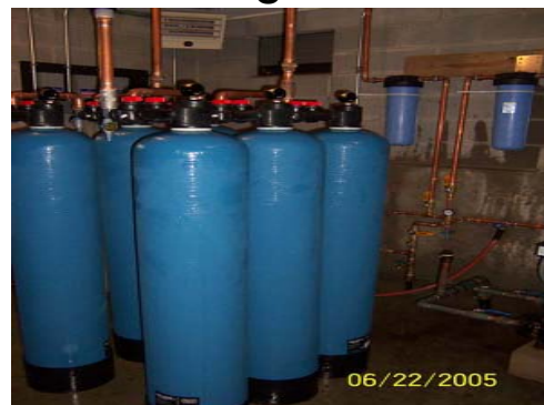
Okanogan's new arsenic water treatment equipment
