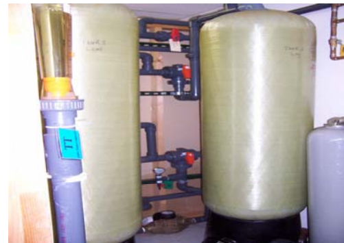
Buckeye's new arsenic water treatment equipment.
