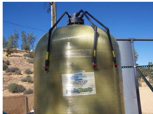
California Water Service Company's new arsenic water treatment equipment
