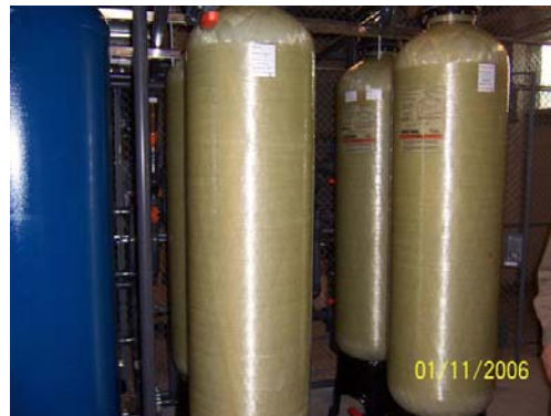
Oregon Institute of Technology's new arsenic water treatment equipment
