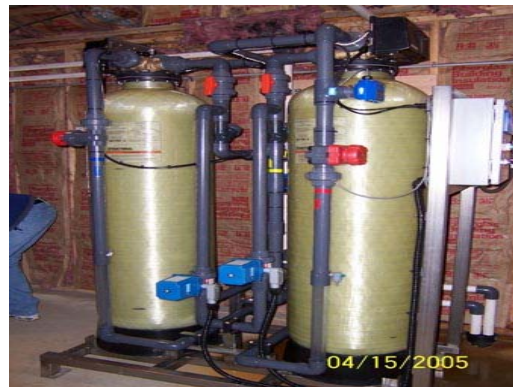
Orchard Highlands's' new arsenic water treatment equipment
