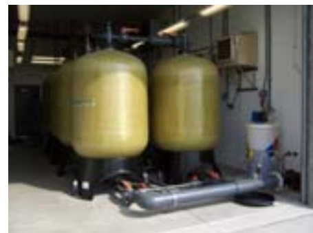
Felton's new arsenic water treatment equipment
