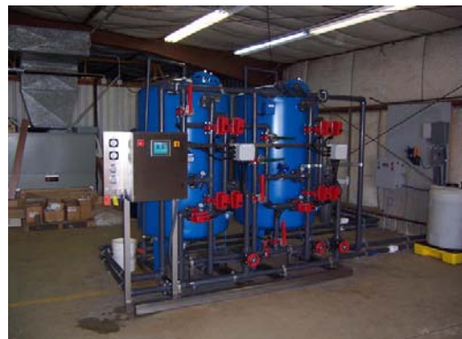
Webb Consolidated Schools' new arsenic water treatment equipment
