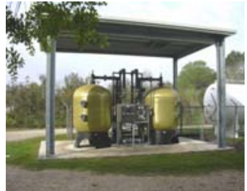
Oak Manor's new arsenic water treatment equipment
