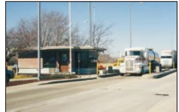
North Platte I-80 mainline WIM sensors
