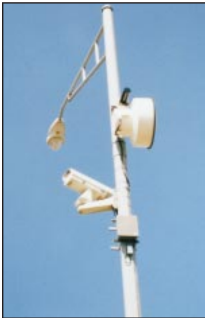
Intersection signal pre-emption device
