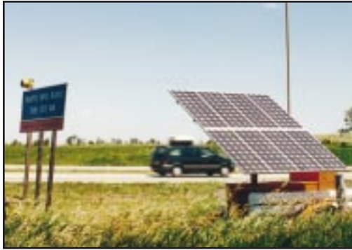
The highway advisory radio and flashing light are powered by a portable array of photovoltaic cells.
