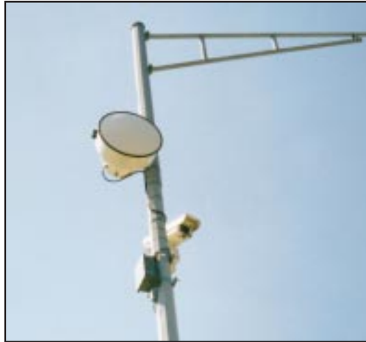
Freeway surveillance camera and antenna at intersection
