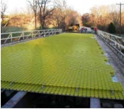
Fiberglass-polymer composites form the core of a renovated bridge deck. Credit: Fabio Matta, UMR.
